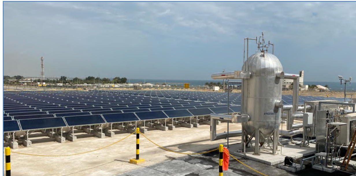
TVP Solar plant in Qurayyah (thermal bloc is on the right of picture)
