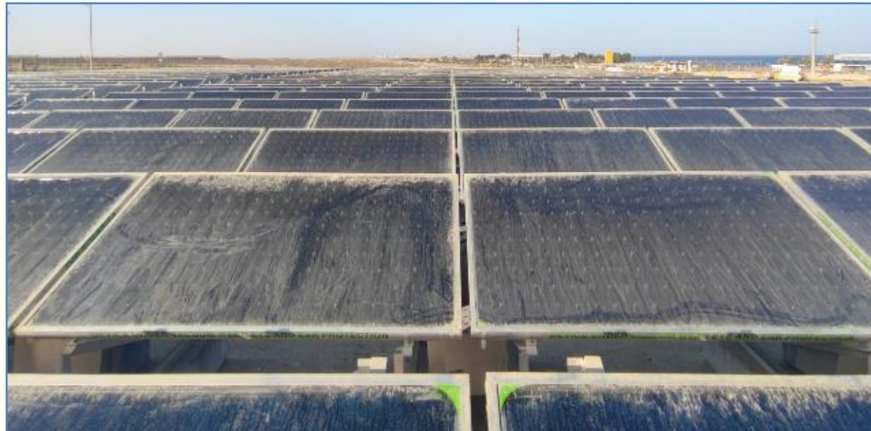
TVP Solar collector in Qurayyah covered with dust and sand
